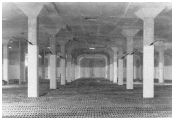
Figure 9.4 – Interior of New Sand Filter at Savannah River Laboratory Before Loading of Sand and Aggregate
