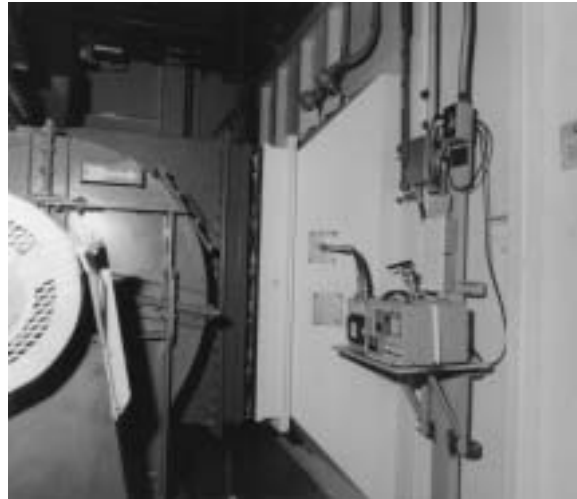
Figure 4.51 – Air Monitor in Exhaust Duct from Plenum
