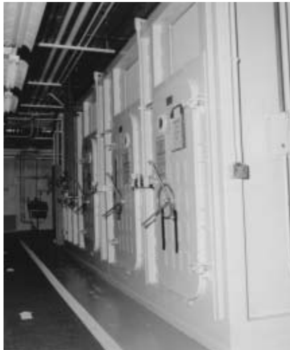
Figure 4.9 – Common Aisle Between Two Man-entry Plenums
