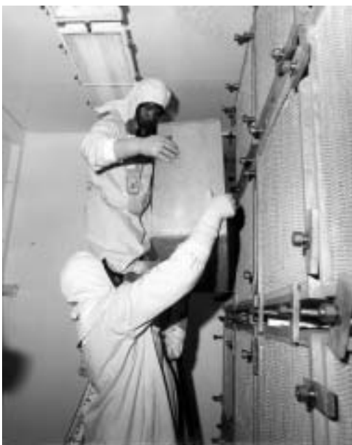
Figure 4.29 – HEPA Filter Mounted on Upstream Side of Mounting Frame Filter Replacement
