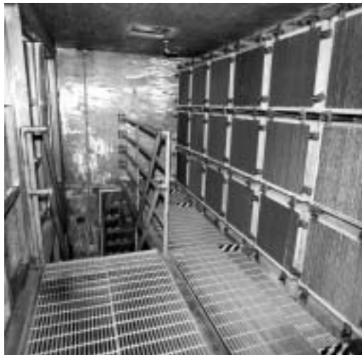
Figure 4.7 – Man-entry Two-Level Plenum (Upper Level Looking at Upstream Side of First HEPA Filter Stage)
