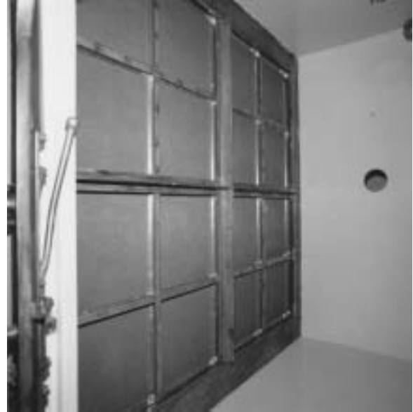
Figure 4.46 – Moisture Separator (Downstream Side)
