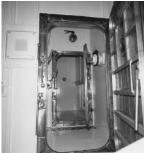
Figure 4.35 – Filter Plenum (Looking from Outside through the Airlock into the Plenum)
