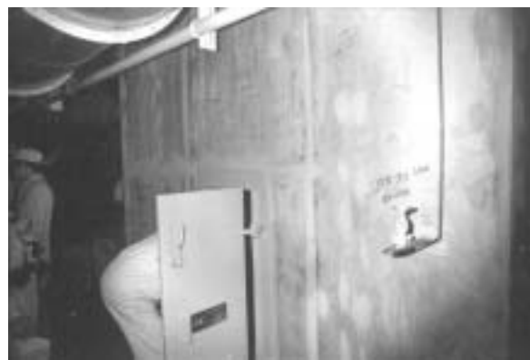
Figure 4.38 – Filter Plenum (Door Bar Style Showing Difficult Access)
