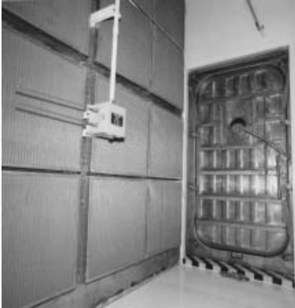
Figure 4.45 – Moisture Separators with Heat Sensor (Upstream Side)
